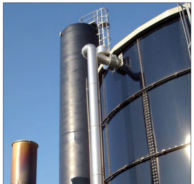
Fig. 1a: General photos of the Bruck an der Leitha biogas plant
